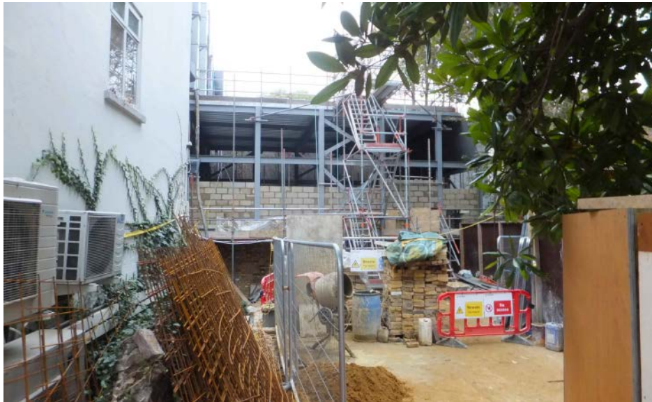
Front elevation in Abbey Road (top) and 'Dolby Atmos studio' under construction in 2016 (bottom).
